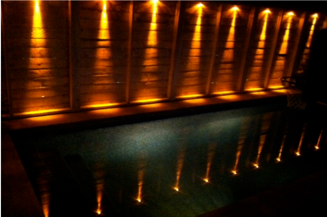
Mounted on top of a fence, effect at night (architectural purpose)
