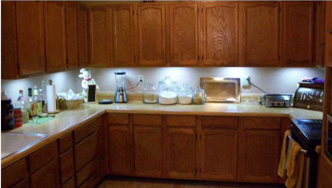
Eight 9-inch LED tubes installed in kitchen
