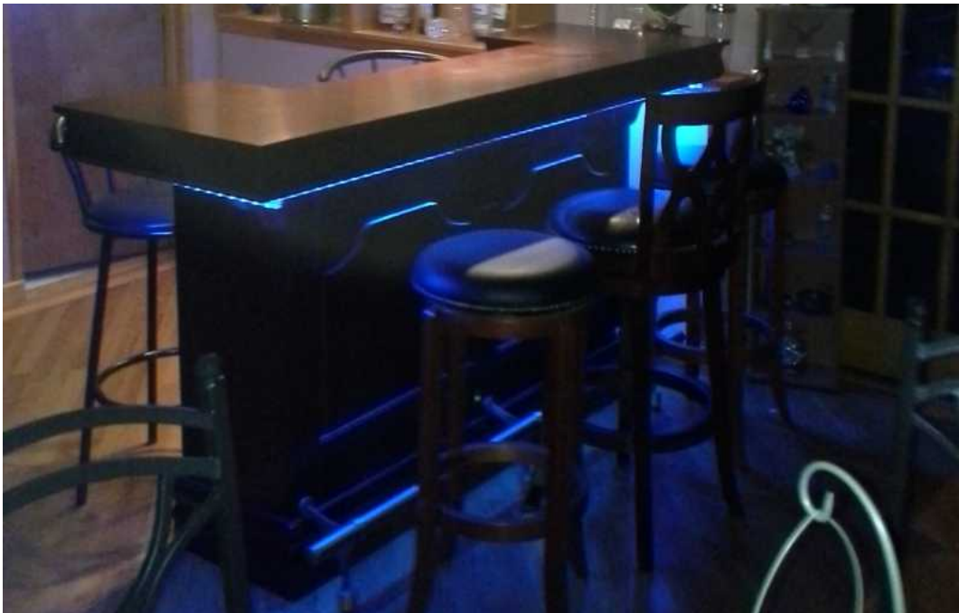
Blue tri-chip tubes installed underside of bar table
